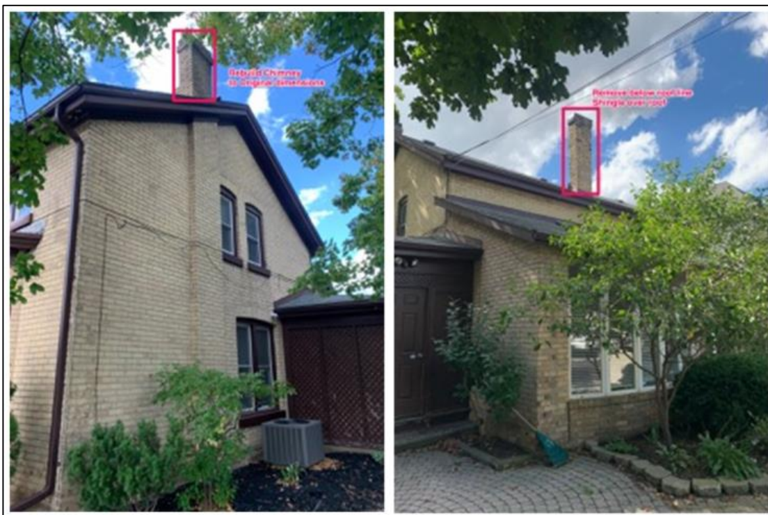
Figure 4: Chimneys at 175 Brant Avenue. Chimney at front-side (left image) to be rebuilt. Chimney at rear (right image) proposed to be removed. Source: Stonebridge Masonry.
