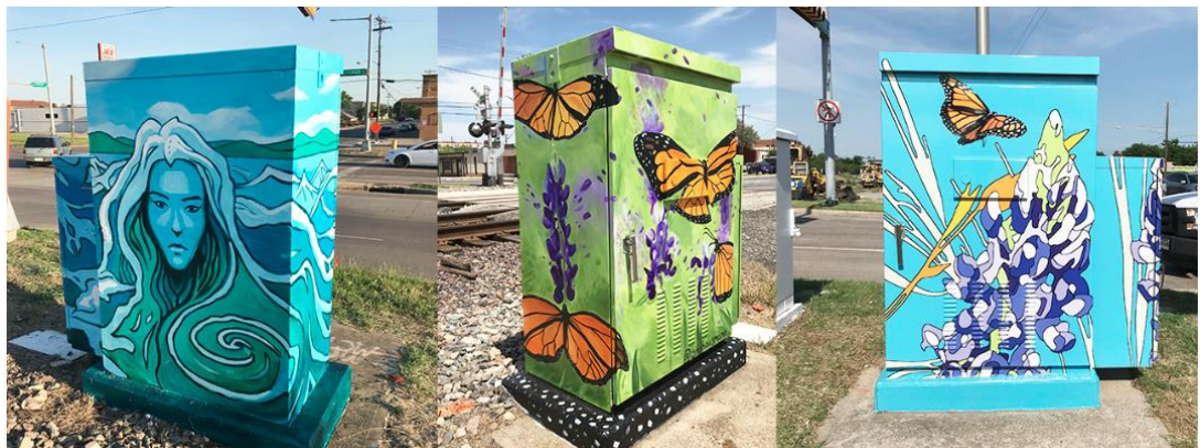
Figure 3 Example traffic cabinets wrapped in mural artwork in other communities.
