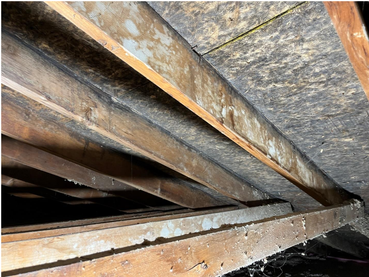
Photograph 1: Mould impacted sheathing and joists found in many of the attics inspected.
