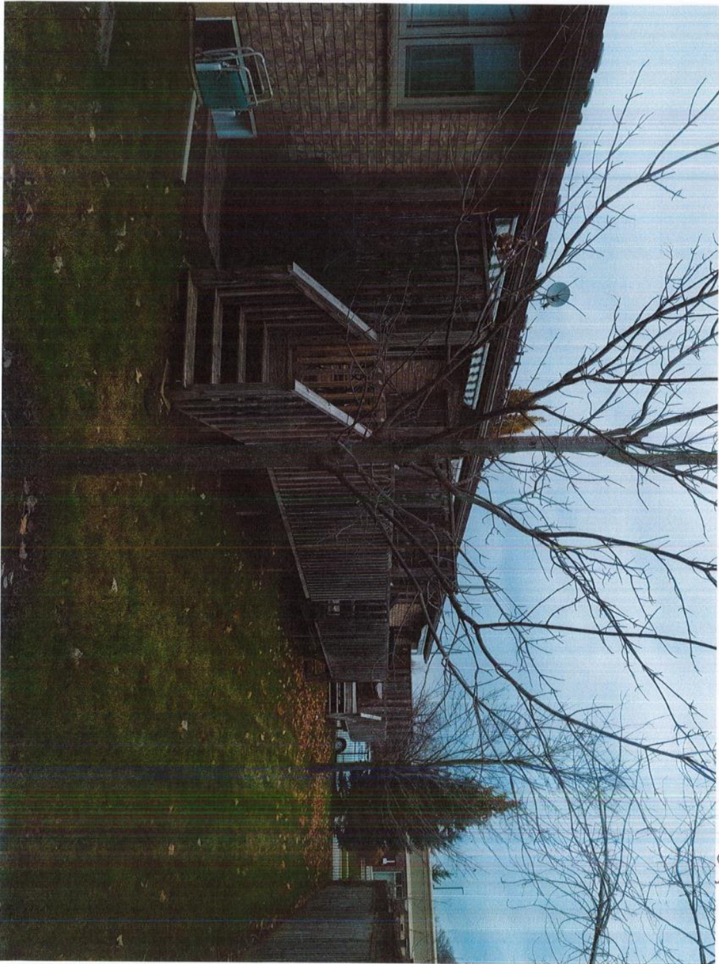
BACK OF UNIT 13 SHOWS MASTER BEDROOM WINDOW AND HEIGHT OF DECK (36" ABOVE BOTTOM OF FENCE,
