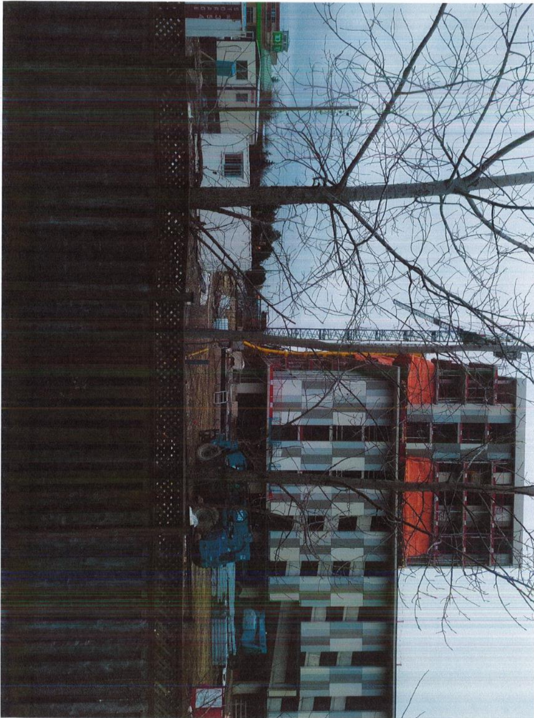
VIEW FROM BACK DECK BUILDING GOING IN ABOUT LITTLE BACK OF BUS LIFT TRUCK AND SIDEWAYS FROM PARADE ENTRANCE TO HIT THE CONSTRUCTION TRAILER
